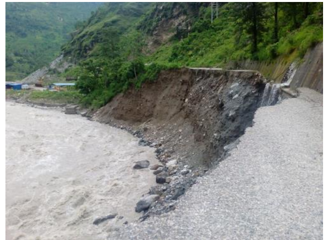
Road damages like these has affected project activities
